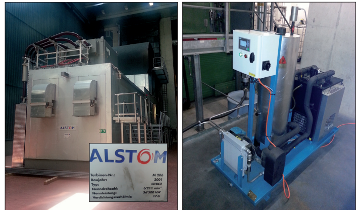
Salzburg AG, Cogeneration Plant, Austria. CJC® Varnish Removal Unit, VRU 27/108 installed at the ALSTOM gas turbine
