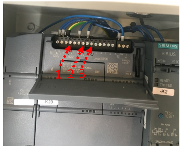
Figure 9: Snap shot of the CMU control box with focus on the external run connections
