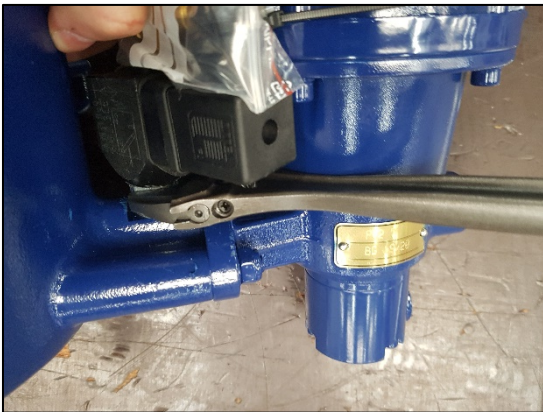
Figure 2: BEFORE - Example of location of the pressure switch at the filter pump pressure side before pressure the filter for CMU connectivity. The pressure switch is reused.
